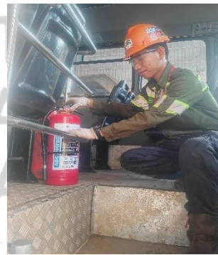
Machine Inspection Program
