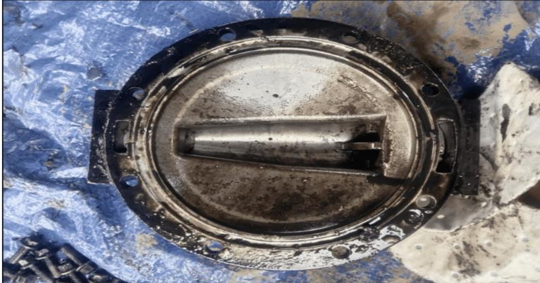
Lampiran 1 Kondisi Fluid Cover Diaphragm Pump Right
