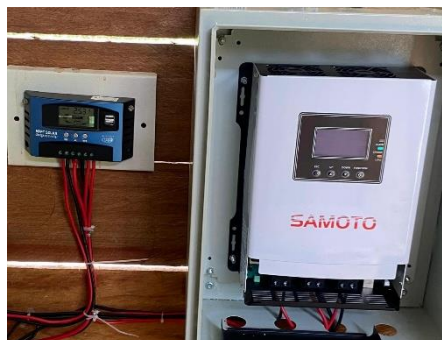
Gambar 2. 5 MPPT &amp; SCC
